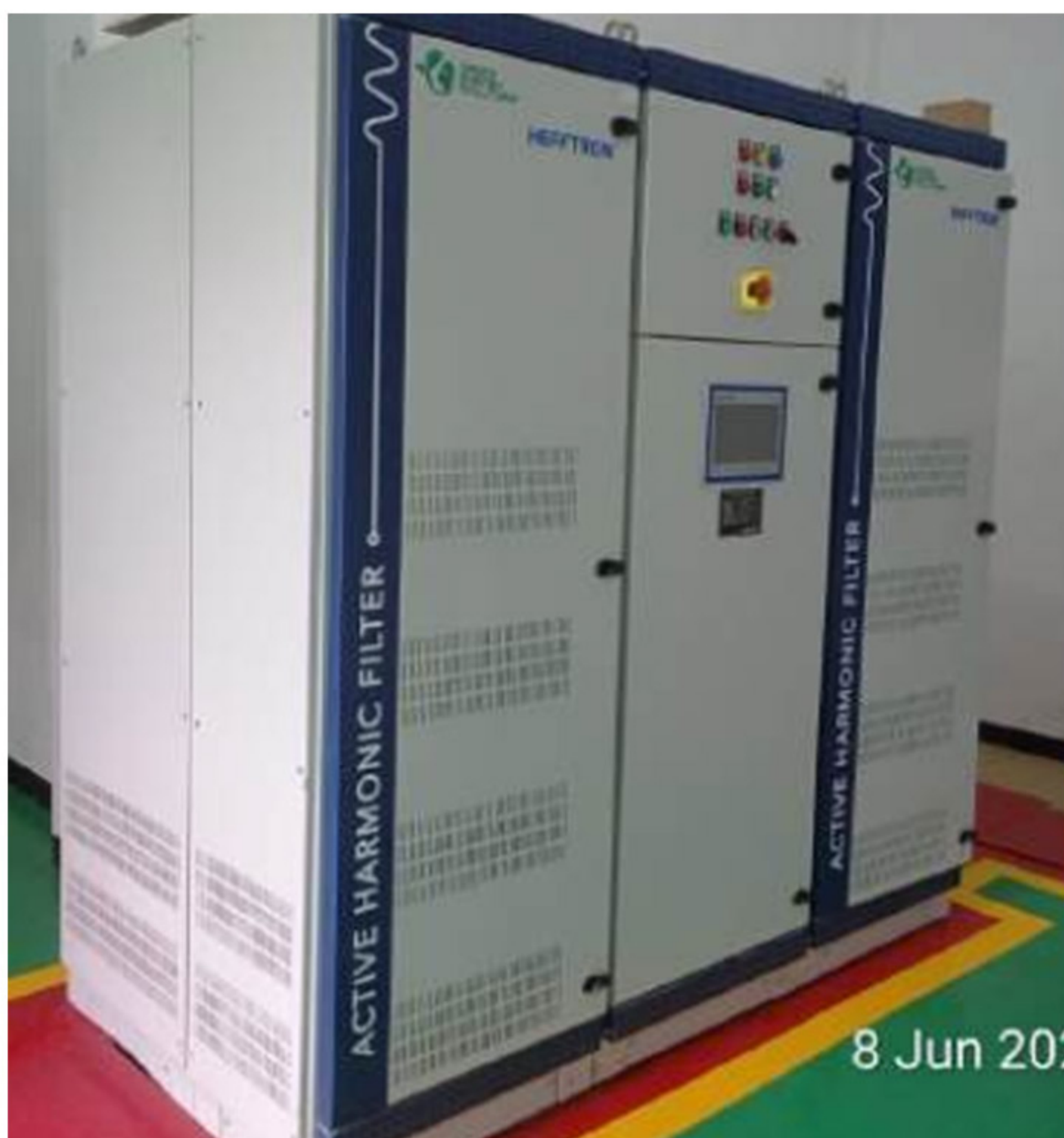
Panel AHF (Active Harmonic Filter) Project IKN Sumbu Timur
