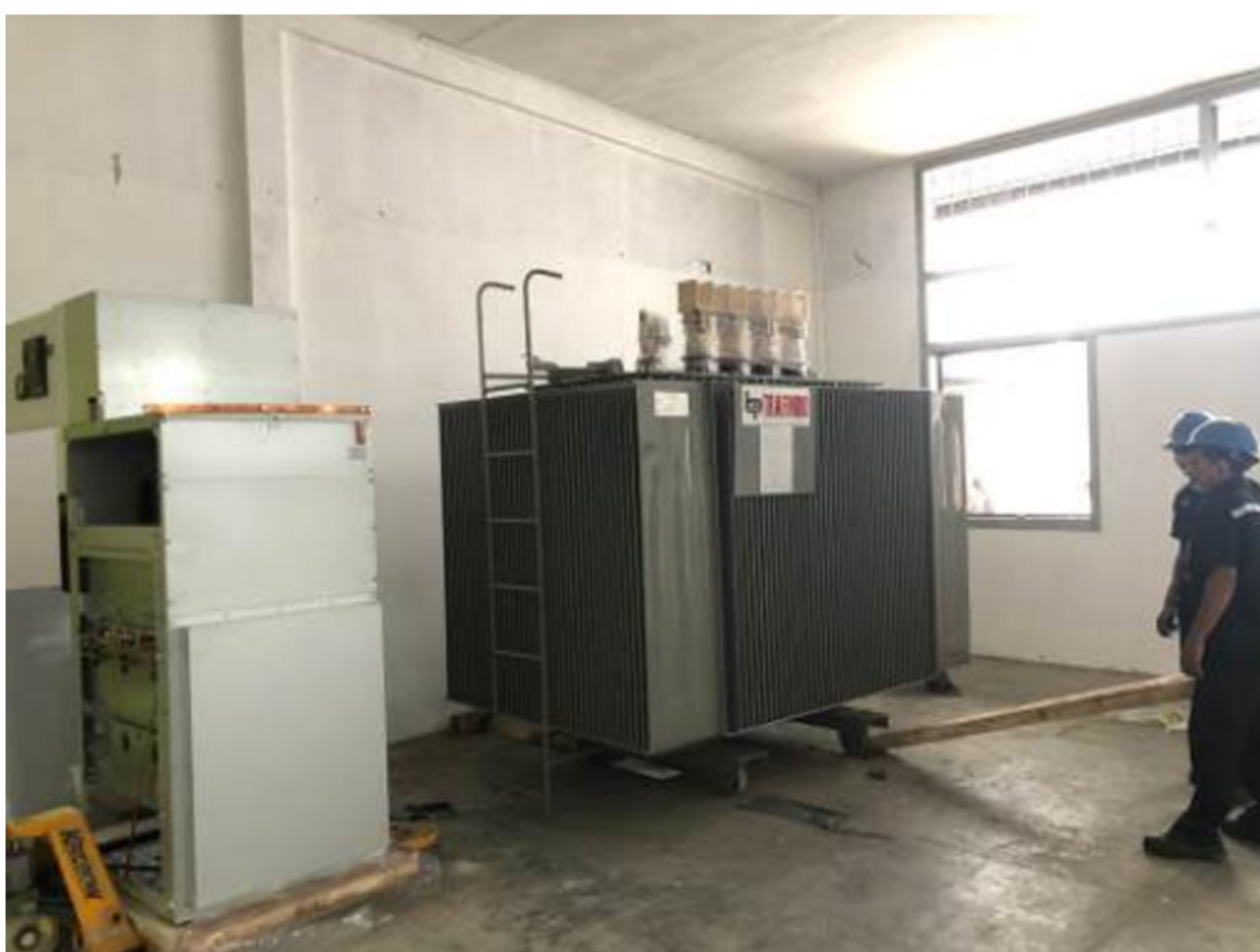
Supplied to Factory PT. Multikabel - Cikande - Serang Banten
