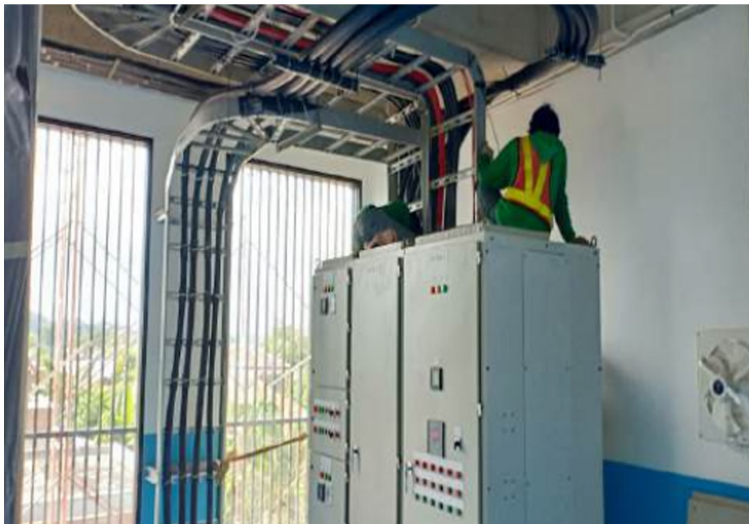
Instal at Hotel Bumi Segah – Kalimantan Timur Owner : PT. Kayan Group / KPP / KPUC
