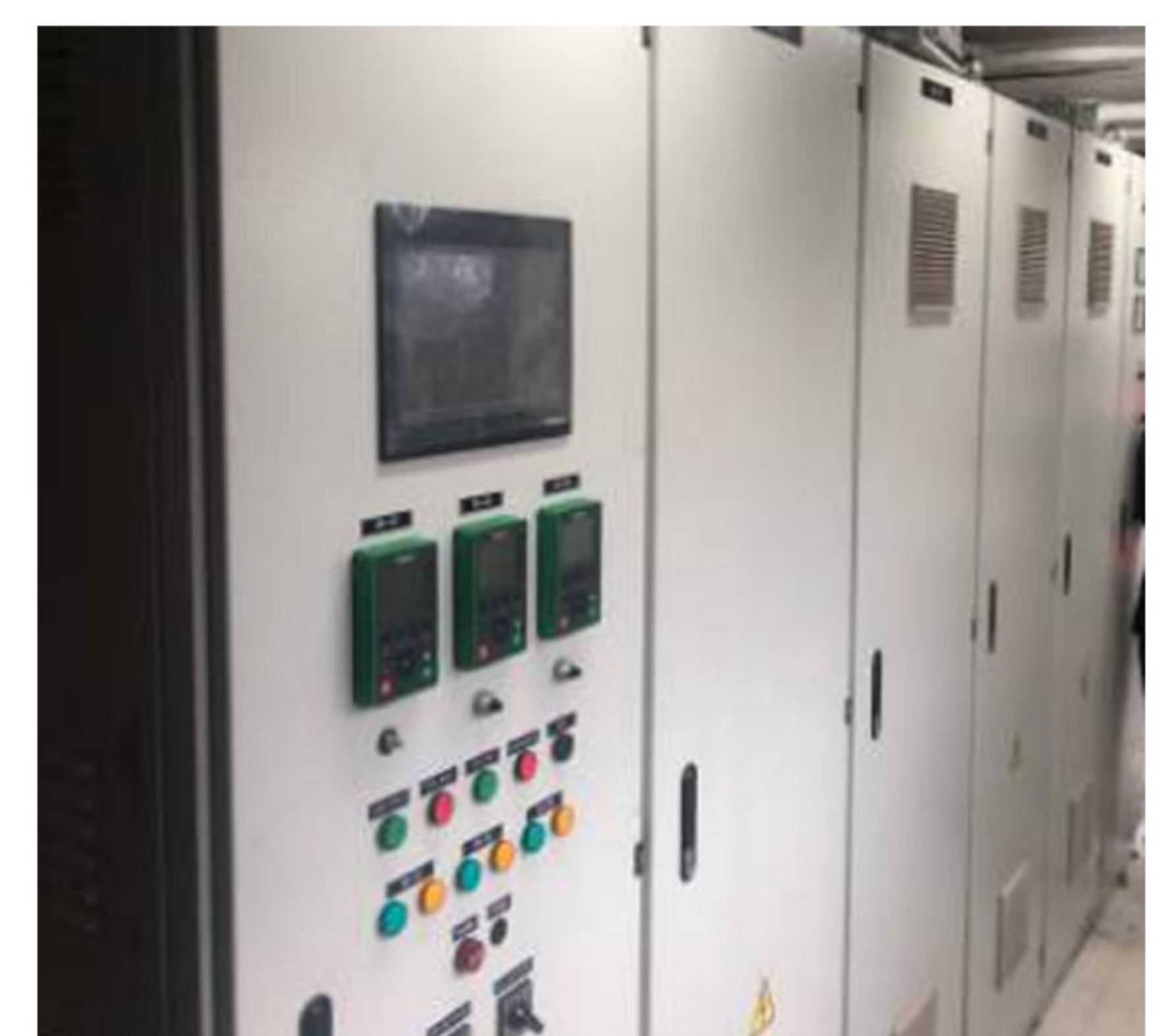
Panel MCC & PLC – for Mining Supply to Project Sungai Puting Port – Kalimantan Owner : PT. Antang Gunung Meratus
